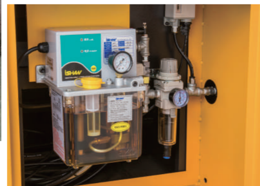
Automatic lubrication unit.
